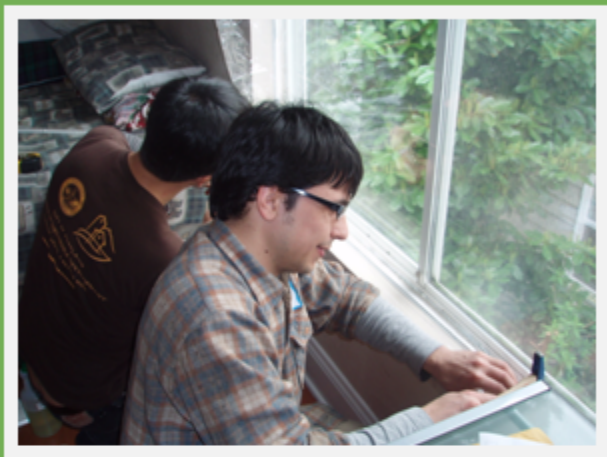
CEP Volunteers weatherizing a client's window with an internally-mounted, reusable storm window kit.
